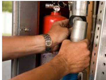
The plant starts automatically when the hose is attached – and stops immediately when the hose is detached.
